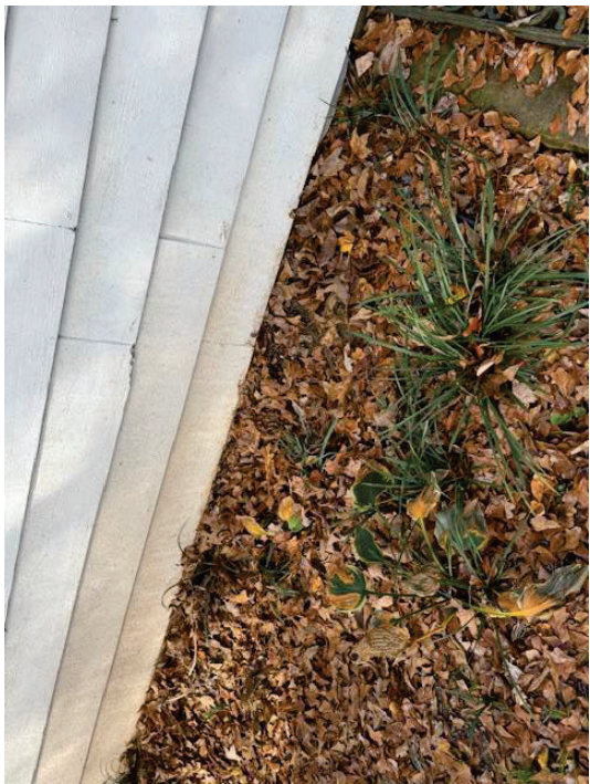
Wall Touches the Ground. No draina
