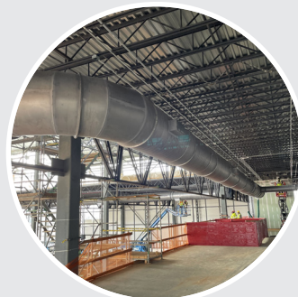
FUNDAMENTAL COMMISSIONING Training Support Facility, Ft. Rucker, AL
