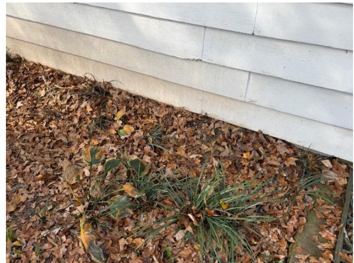
Wall Touches the Ground. No drainage
