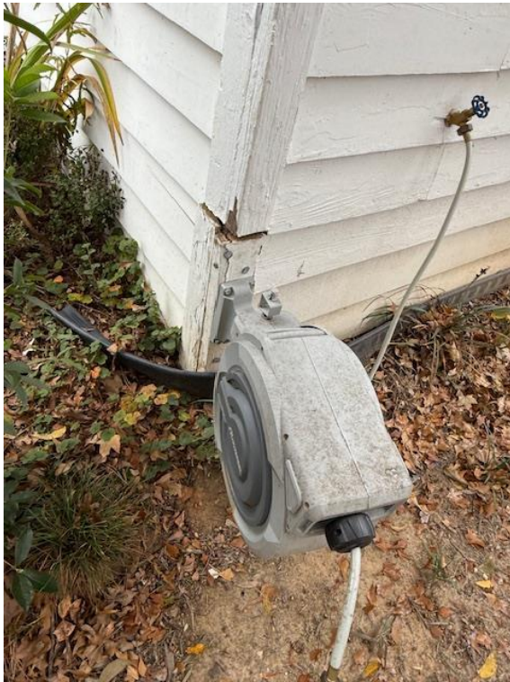
Rotting Wood Siding and Corners
